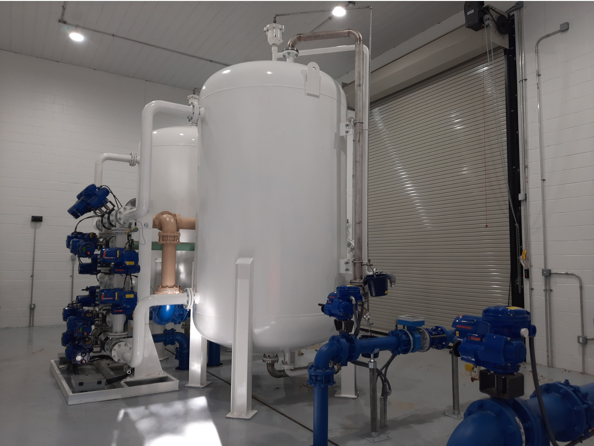
Main treatment and polishing units for Well 11.
