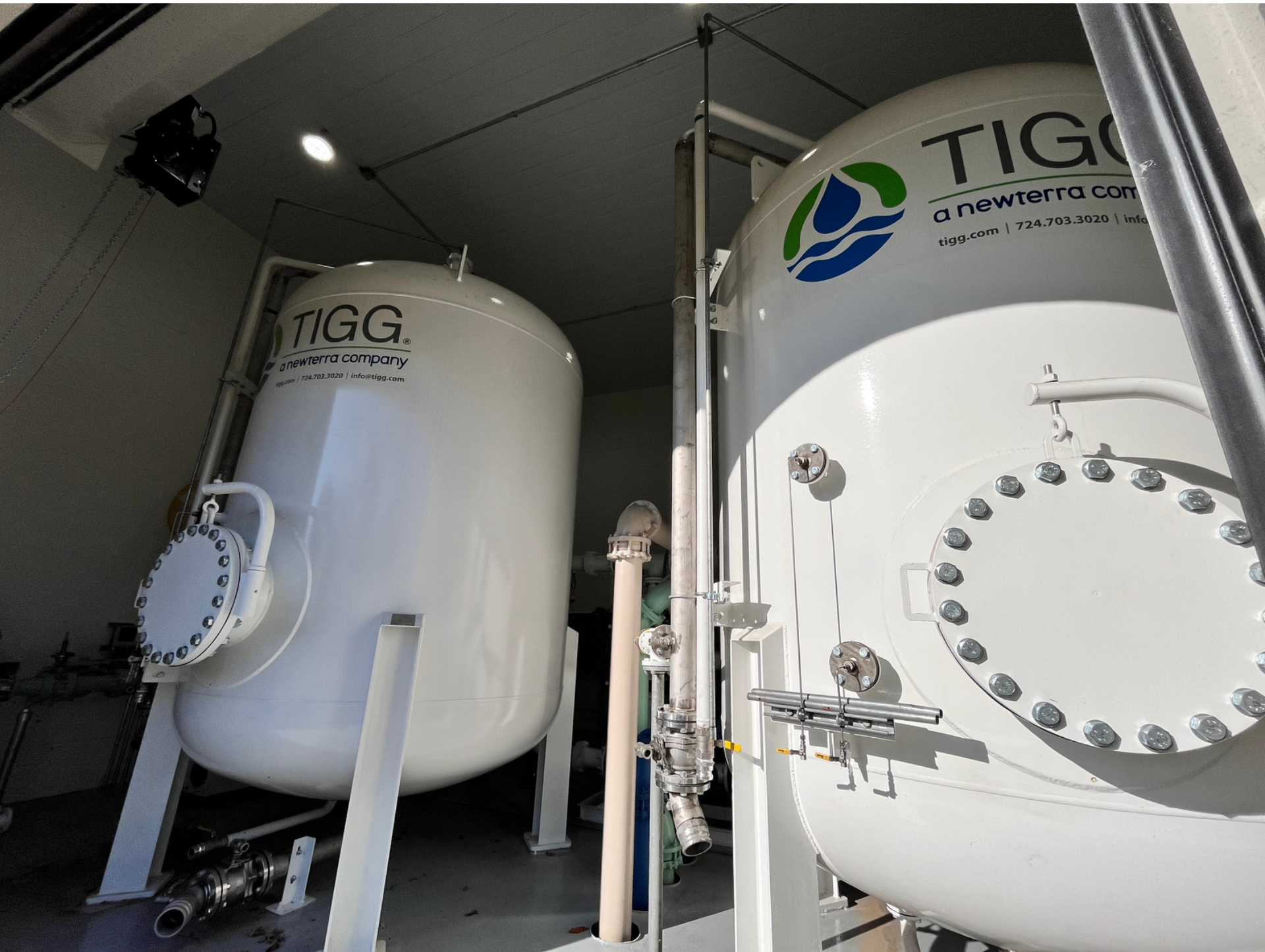
Main treatment and polishing units for Well 3.
