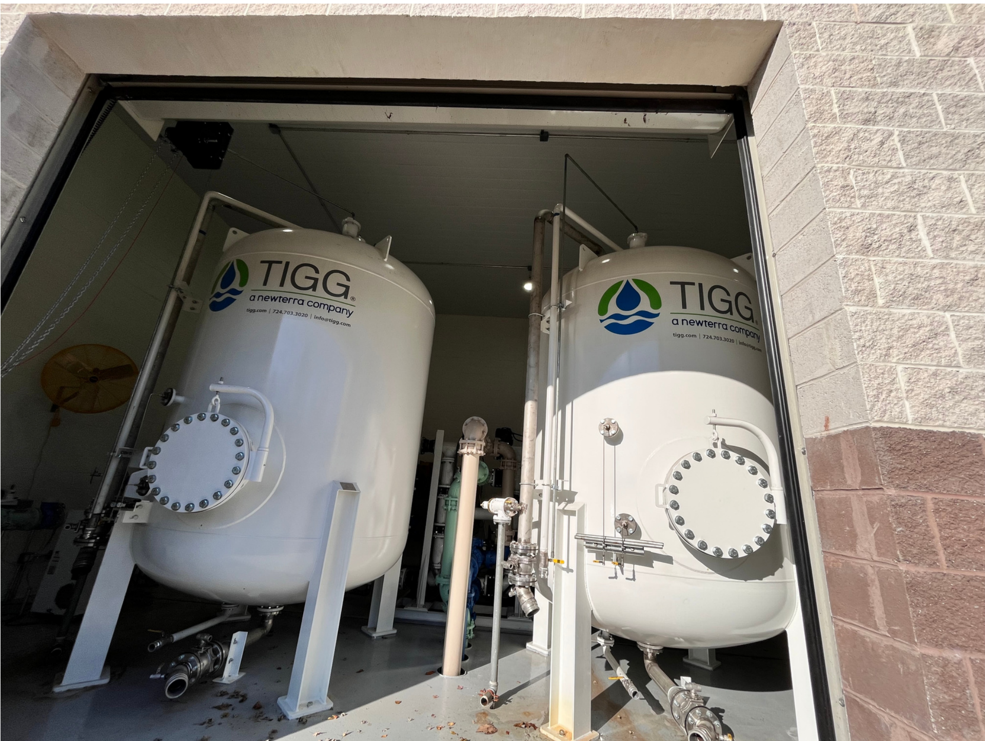
Main treatment and polishing units for Well 3.
