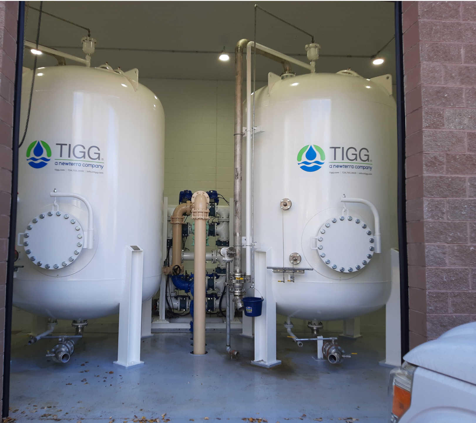
Main treatment and polishing units for Well 5.
