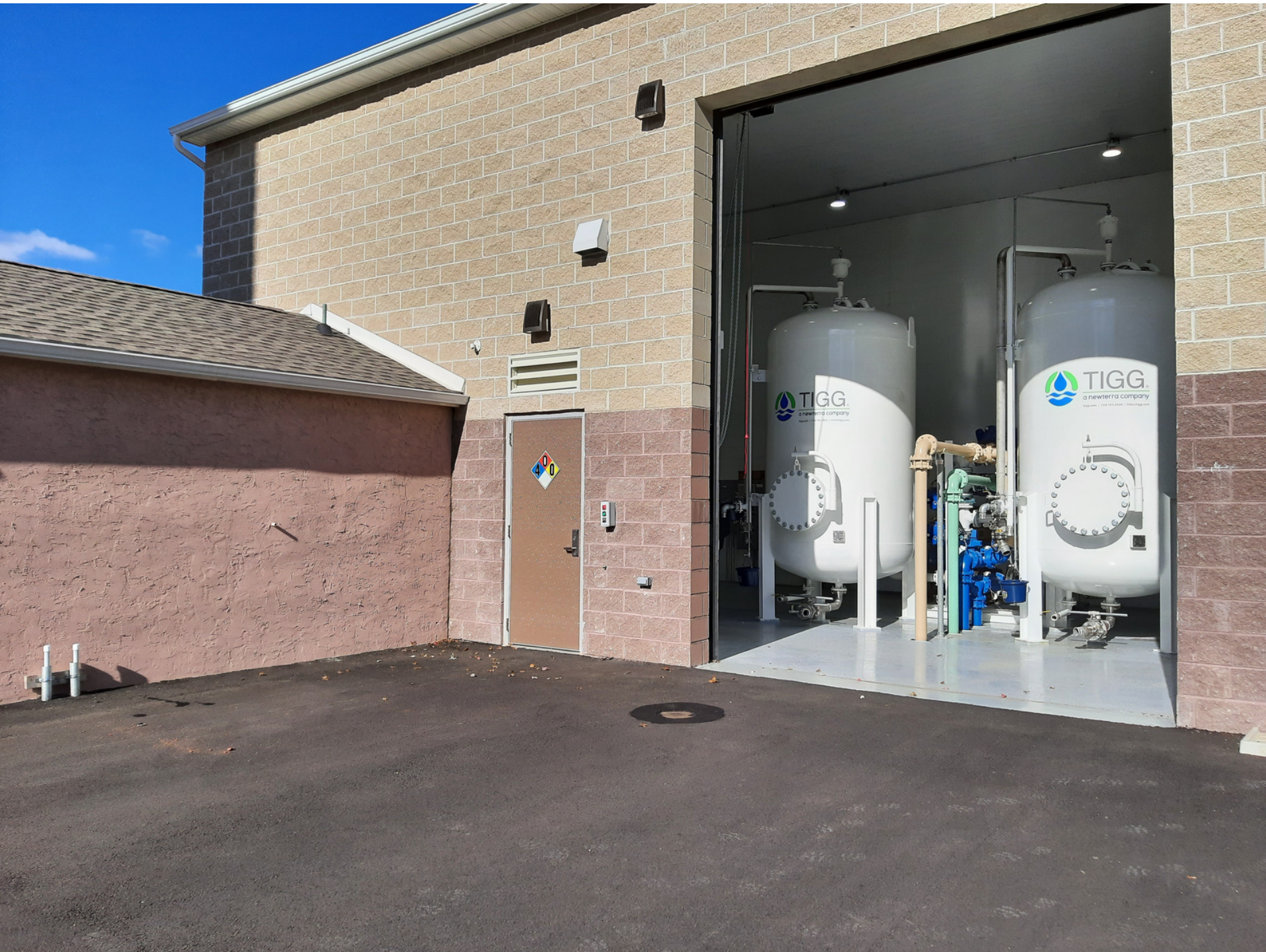
Main treatment and polishing units for Well 8.
