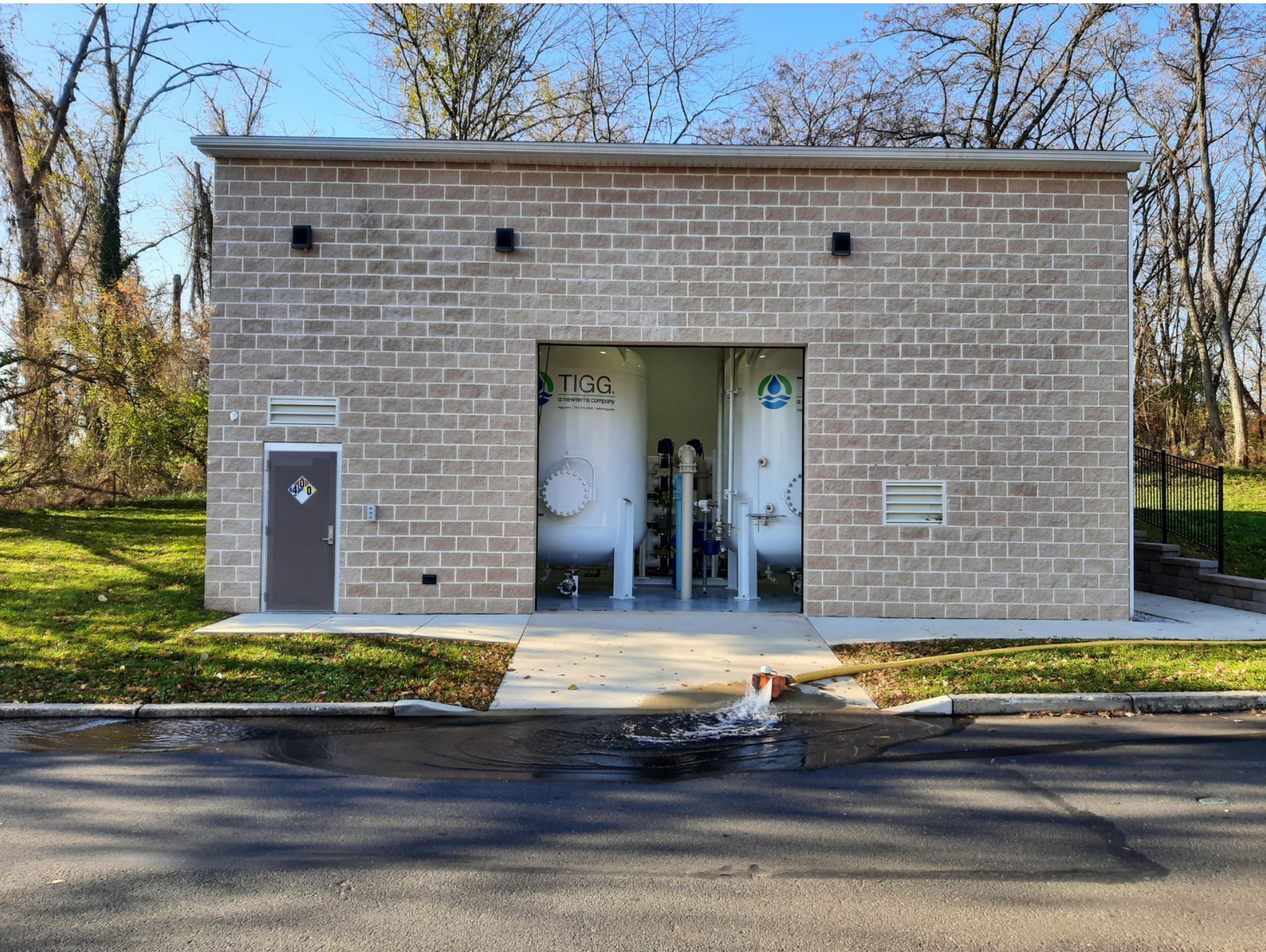
Main treatment and polishing units for Well 9.
